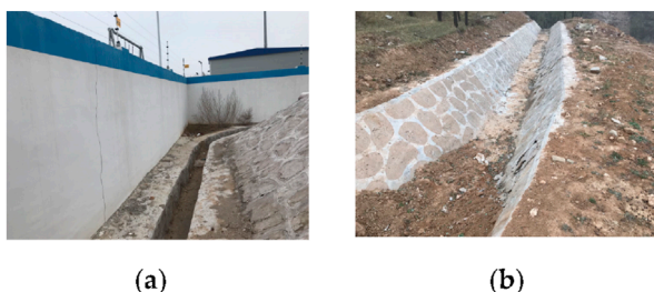
FIGURE 8 Drainage ditch: (a) Drainage ditch at the bottom of the slope; (b) The slope top of the slope intercepts the ditch.
