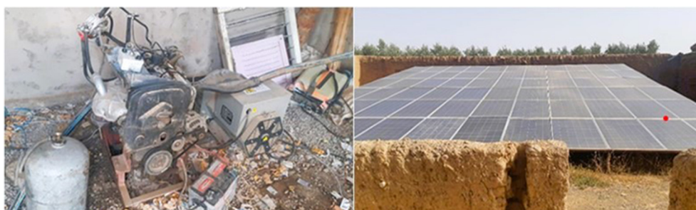
FIGURE 1 Pumping system, installed pv panels. Source: authors.
