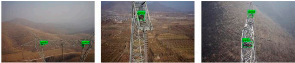
FIGURE 5 Example of a tower defect.
