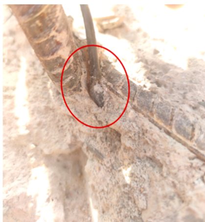
FIGURE 7 Fiber damage caused by chiseling.
