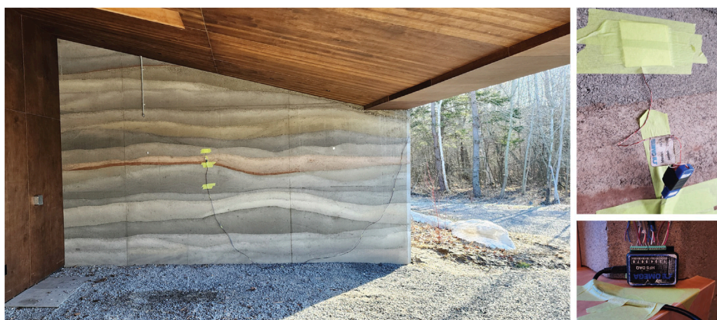
FIGURE 6 Heat flux sensor mounted on the exterior surface of the west-facing wall, with wiring routed through the window frame to connect with the FluxTeg Compaq DAQ system located indoors.
