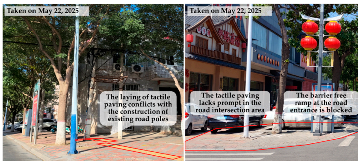
FIGURE 6 The construction of tactile paving is not standardized.
